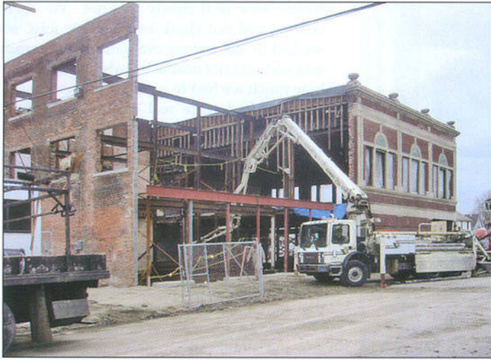
The Monahan Company had to essentially rebuild the entire structural frame and exterior of the back half of Odd Fellows Hall.
